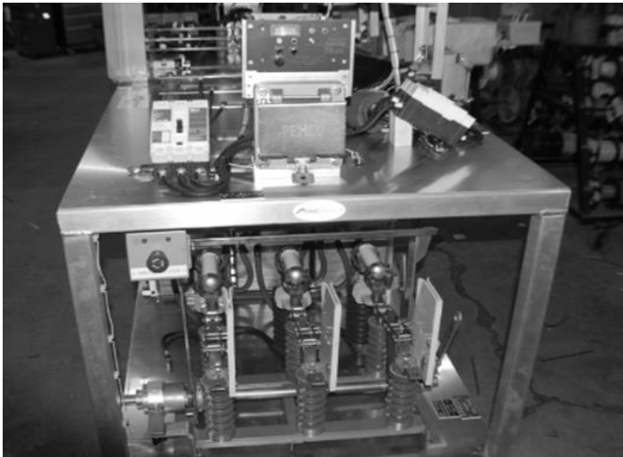
110 Volt Auxiliary Panel
